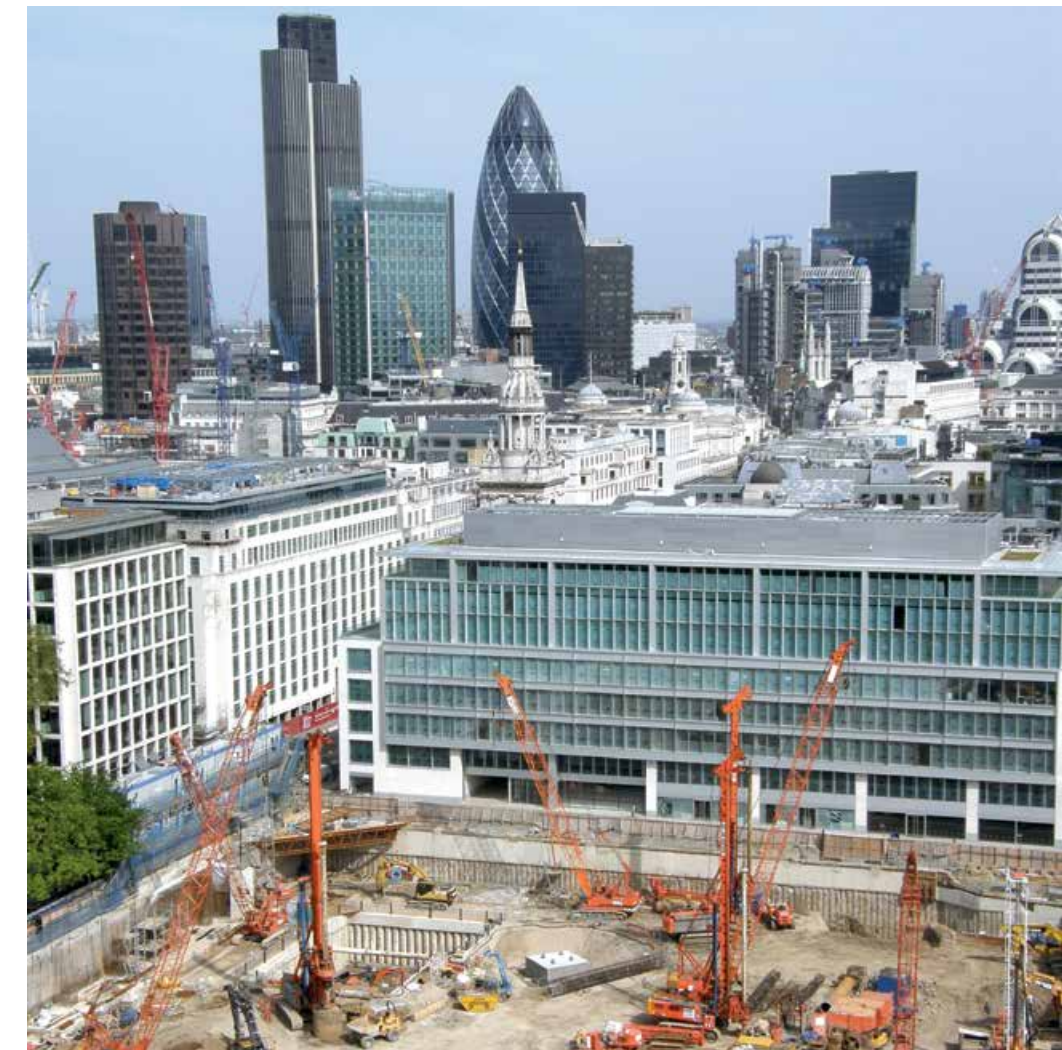
Infill development in central London, UK, makes efficient use of land and creates denser districts to support economic activity and transit capacity.
