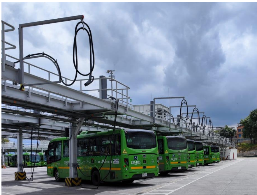
Figure 23. Overhead gantry plug-in chargers for Transmilenio, Bogota - Columbia
