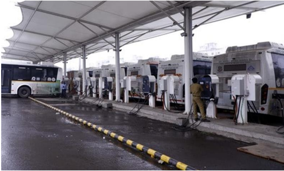
Figure 18. Charging station at an electric bus depot in Pune, India
